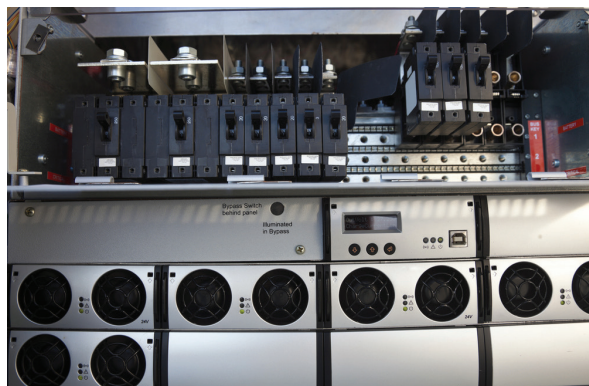
Figure 1. A modular telecommunications power system.
