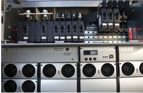
Figure 1. A modular telecommunications power system.
